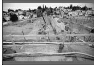
A portion of the construction site of the Highland Hospital Acute Tower... (DEEBAYAVROMSTAFF PHOTO)
