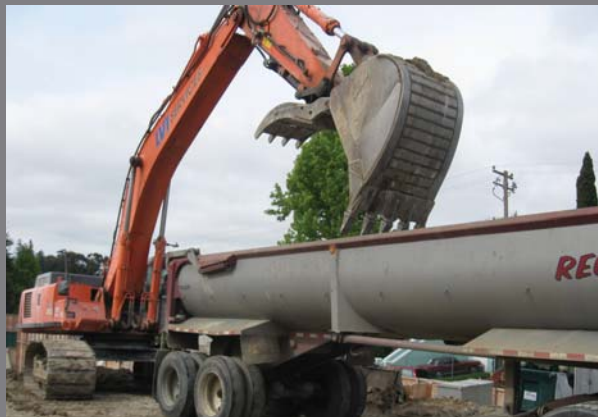
The photo to the right shows the process of trucking construction debris to recycling centers. Currently, over 1,000 truck loads of dirt and demolition debris have been removed from the construction site and recycled.
