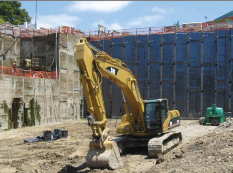
The photo to the left shows the inside of the Specialty Care Clinics Building construction fence. The site is now ready for installation of the foundation to begin.
