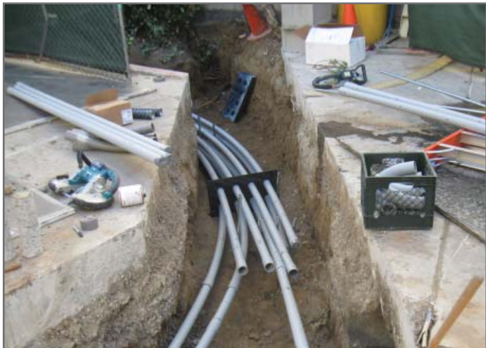
Underground piping between C, D, and F Wings.
